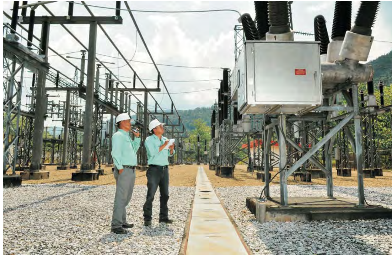
Fasilitas Sambungan Listrik | Power Supply Facility
